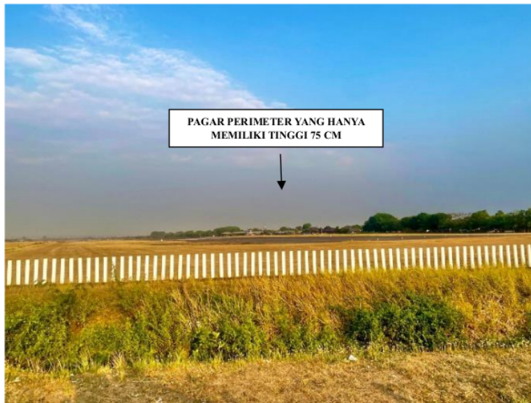
Gambar 4. 1 Pagar Perimeter Area Ujung Runway 08
