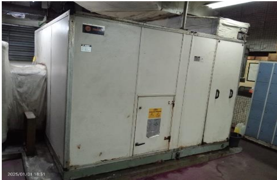
Gambar II. 3 Air handling unit
