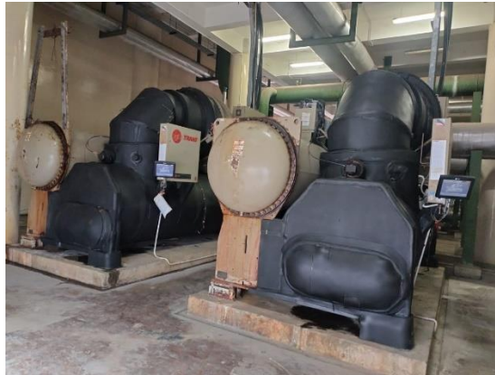
Gambar II. 2 Chiller AC Sentral Bandar Udara Internasional I Gusti Ngurah Rai Bali
