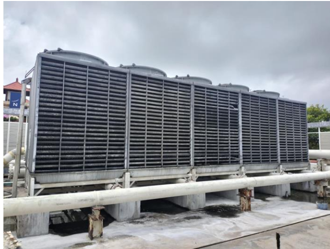
Gambar II. 3 Cooling Tower di Bandara Internasional I Gusti Ngurah Rai Bali
