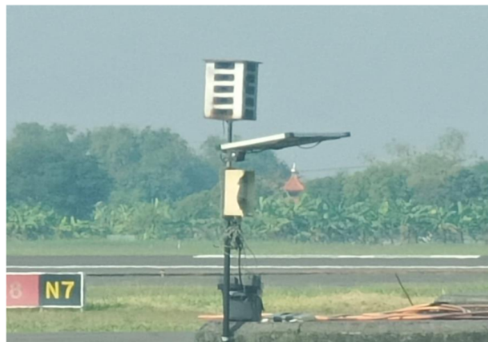
Gambar II. 2 Fasilitas Fix Bird Deterrent (Personel AMC, 2024)
