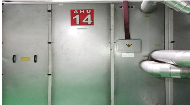
Gambar II. 3 Air Handling Unit
