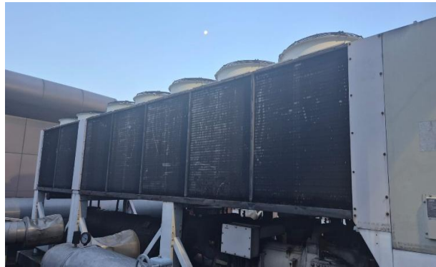
Gambar 2. 1 Chiller Juanda (Sumber: Bandara Juanda, 2025)
